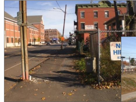
Sidewalk in Poor Condition on S. Side of Monroe Street
