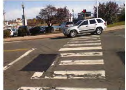
Large Turning Radius On Westbound Approach Of Water Street At Washington Street Encourages High-Speed Travel In An Area With Significant Pedestrian Traffic
