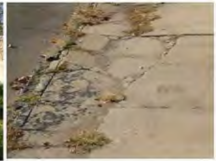
Henry Street Between S. Main And Chestnut Street: Cracked/Crumbling Sidewalks, Lack Of Buffer Between Sidewalk And Roadway
