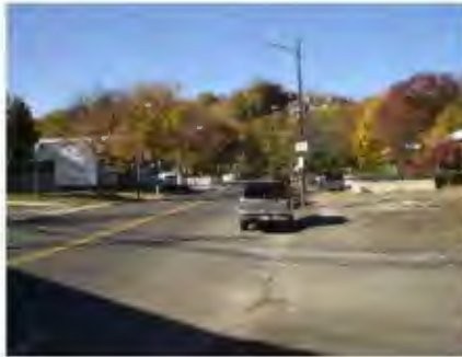
Crumbling And Uneven Sidewalk On The North Side Of Monroe Street Looking West
